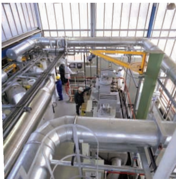
Plant for the cementation of radioactive liquids and sludges
