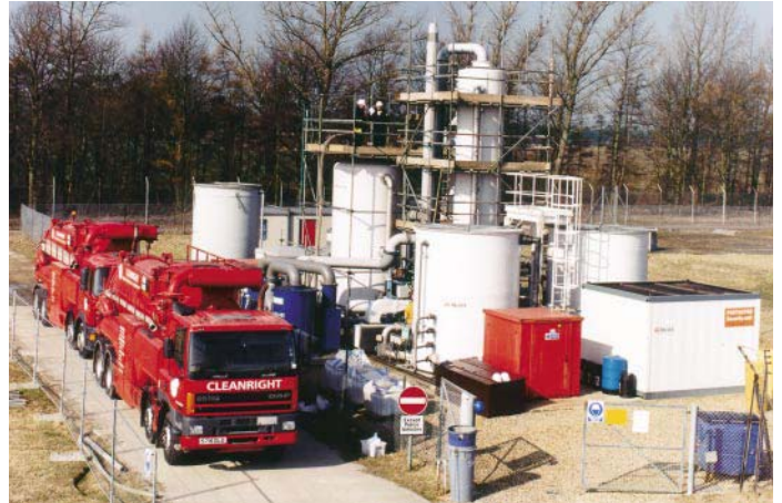
Plant for removal of chlorinated hydrocarbons from groundwater
